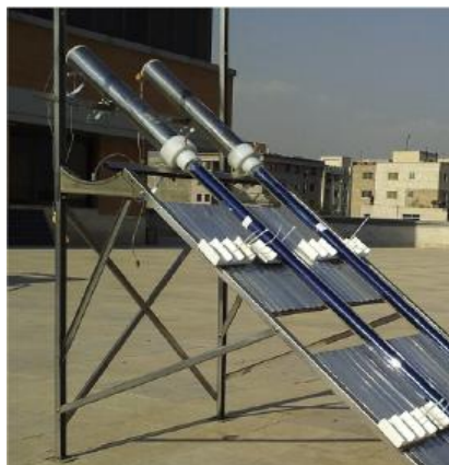
condenser mounted axially above with evacuated tube condenser (Shafii et al. 2016)
